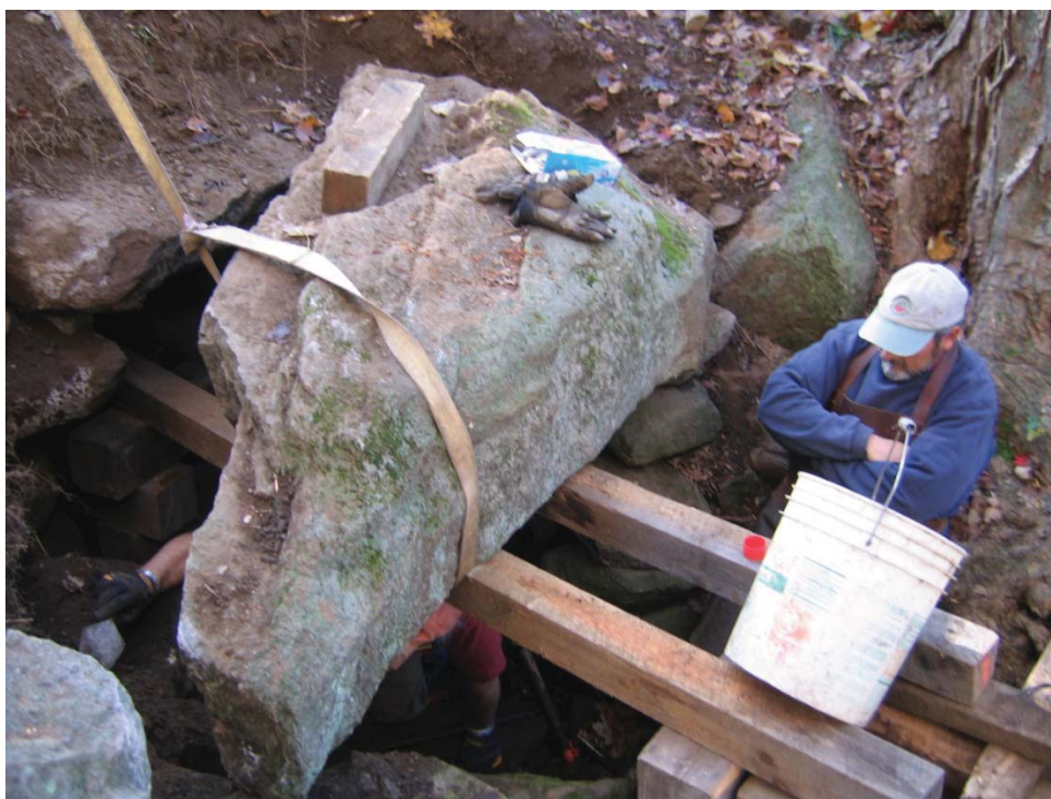
Plate 35. In-situ lintel secured with a strap and supported by cribbing, view south; note large gap behind lintel caused by loss of ceiling boulder and forward shifting of the lintel.
